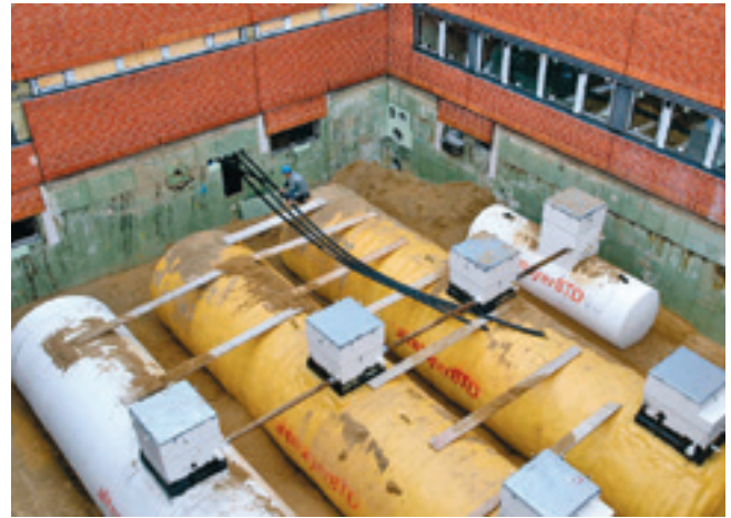
The tanks were lifted over the 4-storey building into the inner courtyard by a 100 tonne load crane
