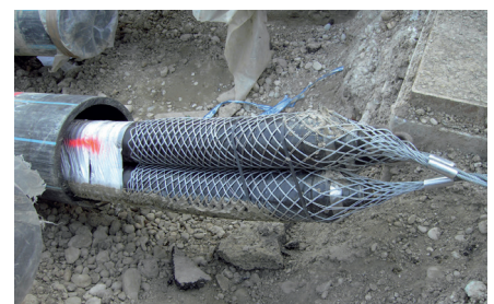
CASAFLEX pipe leaves the jacket pipe after a continuous distance of 190 meters.
